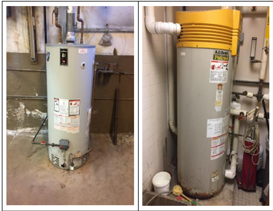
Image 5 – Hot Water System
